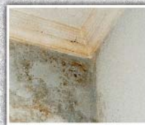
Water ingress harms interiors
