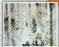
Dampness leads to health problems
