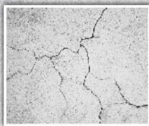
Cracks develop over time
