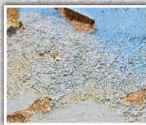
Exposed to weathering
